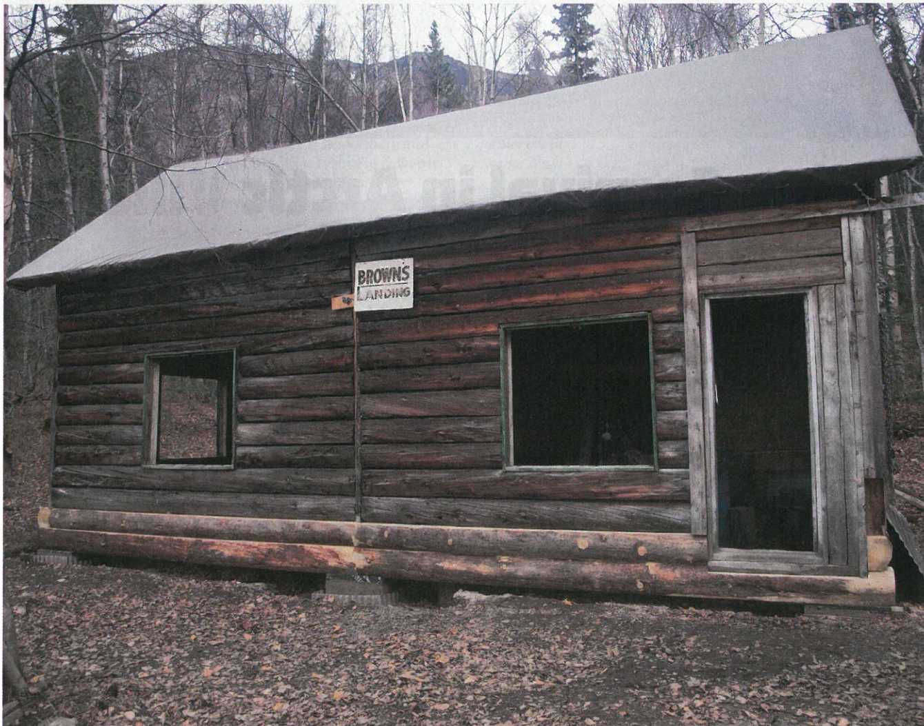
In the fall of 2015, all the new logs were in place. A new roof, floor, installation of windows, and door repair were projects for future seasons.
