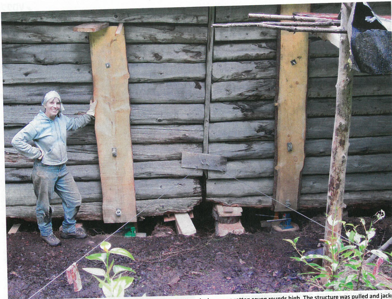
Anne Coray stands along the north wall of Brown Carlson's cabin where the logs were rotten seven rounds high. The structure was pulled and jacked into a level position before the logs were replaced.
