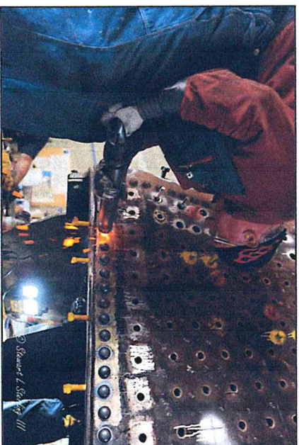
"Hot Riveting" - a nearly forgotten art - is used to reassemble the new firebox into the boiler.
